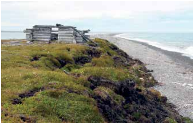
Figure 8. Inuvialuit cabin at Nunaluk Spit, Ivvavik National Park, Yukon coast in 2012; as of 2015 the cabin is undercut but the bluff slope.
