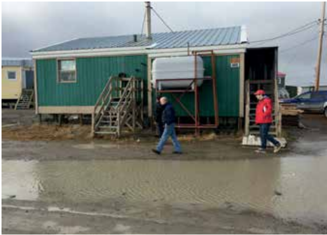
Figure 6. Poor drainage around housing is a health concern and potential cause of differential thaw subsidence and foundation instability in Arviat.
