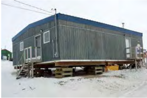
FIGURE 12. Raised building foundation on timber cribs to minimize the impact of the building's heat on underlying permafrost, Taloyoak, NU.
