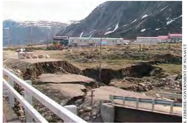
FIGURE 9. Damage to the Duval River bridge in Pangnirtung, NU after a major rainfall flood in June, 2008. The bridge was rendered unusable, which separated important community facilities, and disrupted water and sewage transport until it could be replaced.
