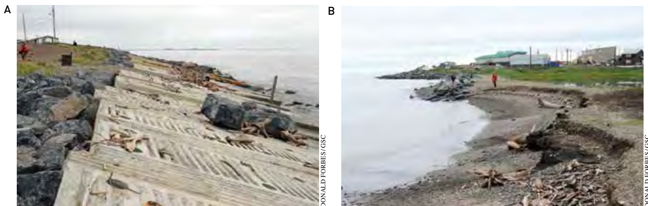
FIGURE 30. (a) Concrete mats installed as shore protection at Flagstaff Point, Tuktoyaktuk, NT, 2012, looking south. (b) Backshore peat exposed in beach scarp on South Spit, Tuktoyaktuk, 2012, reflecting landward rollover and migration of the spit (see Figure 18). View looking north to the Elders’ home and other structures built seaward of it on the former school site. Rubble block shore protection can be seen at the point and extends south along the spit, with erosion and spit migration beginning at its southern end in foreground.
