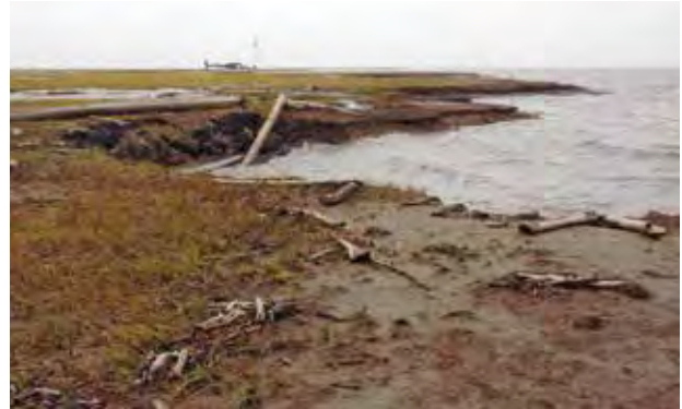
FIGURE 17. Navigation aid tower at Tent Island, YT, 2010 on the west side of Shallow Bay, one of the most rapidly eroding parts of the Mackenzie Delta front. Shoreline retreat here has at times exceeded 20 m year -1 . The Decca navigation station at which two lives were lost here in the September 1970 storm would be far out in the water today.
