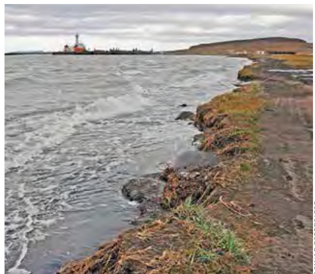
FIGURE 29. Shoreline erosion and washover sand west of the port facility at Kugluktuk, NU, 2009, looking east, with tug and barge in port. Offshore breakwater visible at left and high ground in the outer Coppermine Delta just visible in the background.
