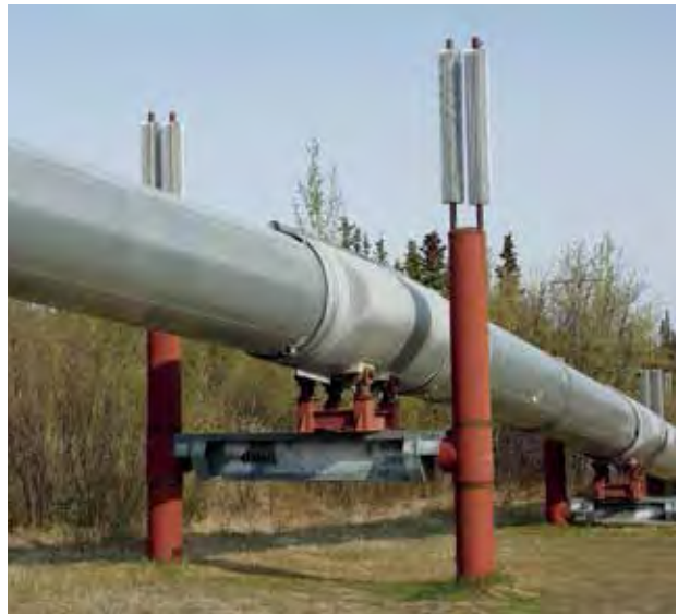
FIGURE 16. Construction approach used on the Alaska Pipeline in central Alaska in permafrost terrain. The pipeline carries oil heated to 49°C to reduce viscosity and allow movement over the length of the route. The pipe is suspended on a pedestal with thermosyphons to minimize ground thaw. Additionally, the pipe is able to move laterally on a sliding block to accommodate thermal contraction and expansion of the pipe during seasonal climate fluctuations.
