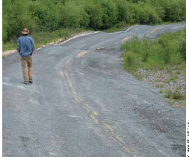
FIGURE 14. Severe road heaving on an abandoned portion of the Ingraham Trail, east of Yellowknife, NT. This example shows how quickly roads built on ice-rich permafrost can degrade.
