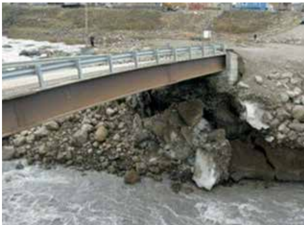
FIGURE 9. Damage to bridge foundation in Pangnirtung resulting from the down cutting of the river bed by thermo-erosion.
